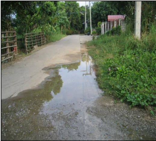
Figure1 Broken pipes in the area
