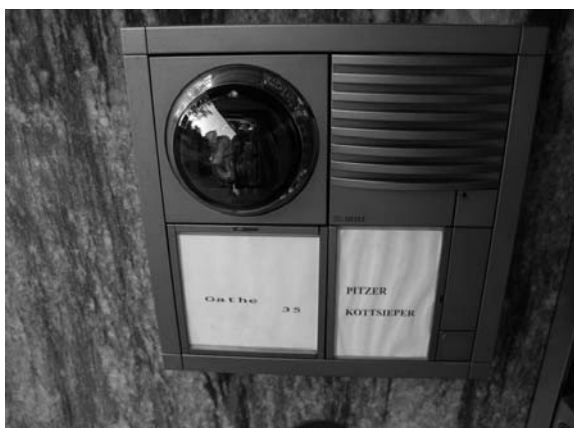
Fig. 3: Digital monitoring device in entrance
