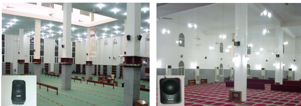
Figure 61. Two different mosques with an installed distributed sound system
